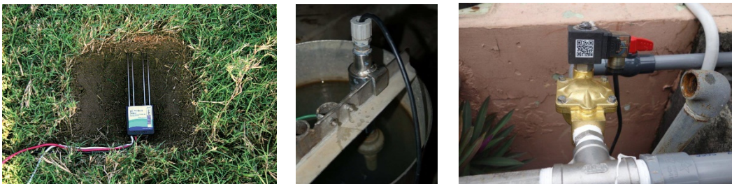
Figure 5 Soil Moisture Sensor, EC (pH) Sensor and Solenoid water valve installation
