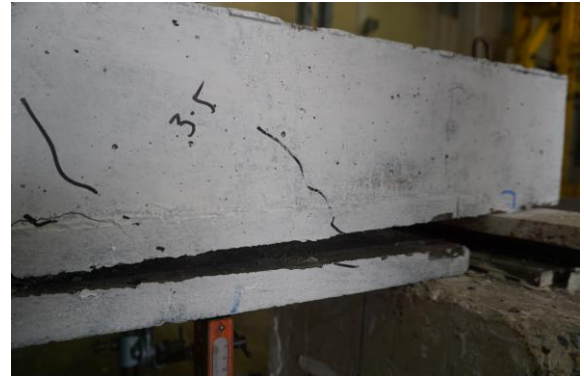
Figure 19. Jacketing separation in beam MEAS-10
