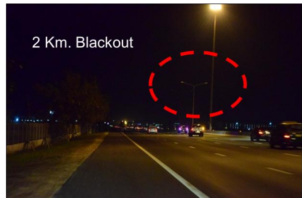
Figure 11. Problems on lighting.
