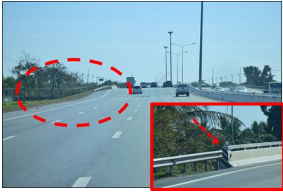
Figure 6. Problems on crash barrier: end treatments and connection
