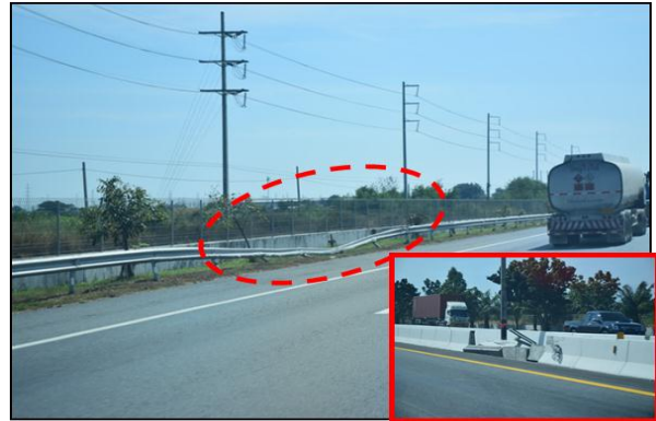
Figure 10. Problems on roadside hazards: crash barrier
