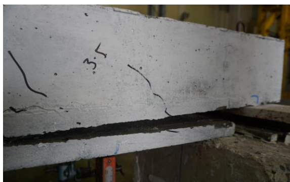
Figure 19. Jacketing separation in beam MEAS-10
